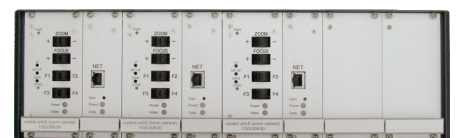
6-camera rack equipped with three camera modules and three video servers
